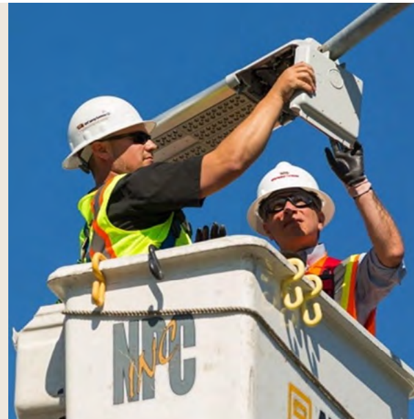
On Mar. 28, 2017, Mayor Ethan Berkowitz joined an ML&P crew to install a new LED street light and 'smart' controller node. (Photo credit: Wayne Johnson, ML&P)
