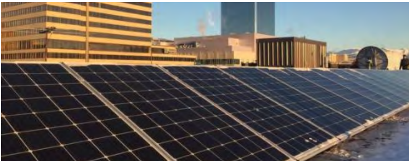
25-kW solar installation on a commercial building in downtown Anchorage. Photo credit: Arctic Solar Ventures
