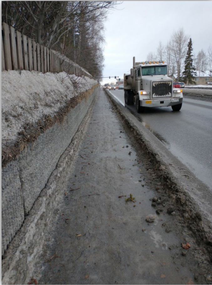
Sidewalks are narrowed and closer to traffic
