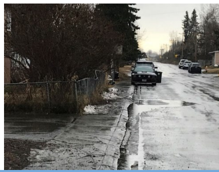
Parked car and remnants of plowed snow on a cracked, broken sidewalk.
