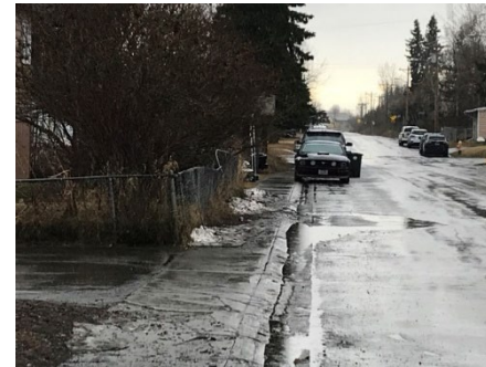
Parked car and remnants of plowed snow on a cracked, broken sidewalk.
