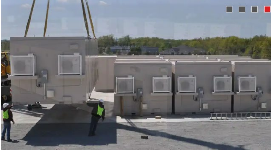
Figure 4. Example installation of ARC vault similar to JBER Foundry site.
