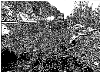
Alaska Railroad crews inspect and repair stretches of track rendered impassable after Friday's earthquake.
