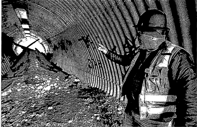
DOT project engineer Jason Badley points out damage to a pedestrian underpass beneath Eagle River Loop Road on Saturday. During the Friday morning earthquake, an 8-inch water main broke, causing the damage. LONNIE HOLMES / APH
