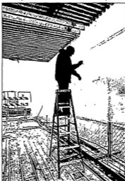
Ritchey Walker of Dowland Construction dangles a plumb bob to make sure pins are properly aligned in the floor and ceiling to attach panels after cement is poured for the floor at the Anchorage Museum Transit Transfer Facility.
