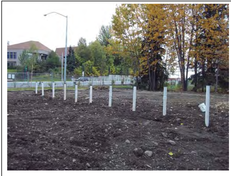
Photo 12: Facing northwest, the VES array was completed with vertical riser pipes. Rubber slips caps were installed on the north array. (9/16/2011)
