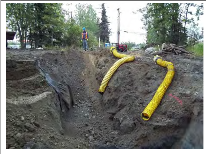
Photo 9: Facing north, fans provided ventilation during the excavation to reduce organic vapor concentrations. (9/2/2011)
