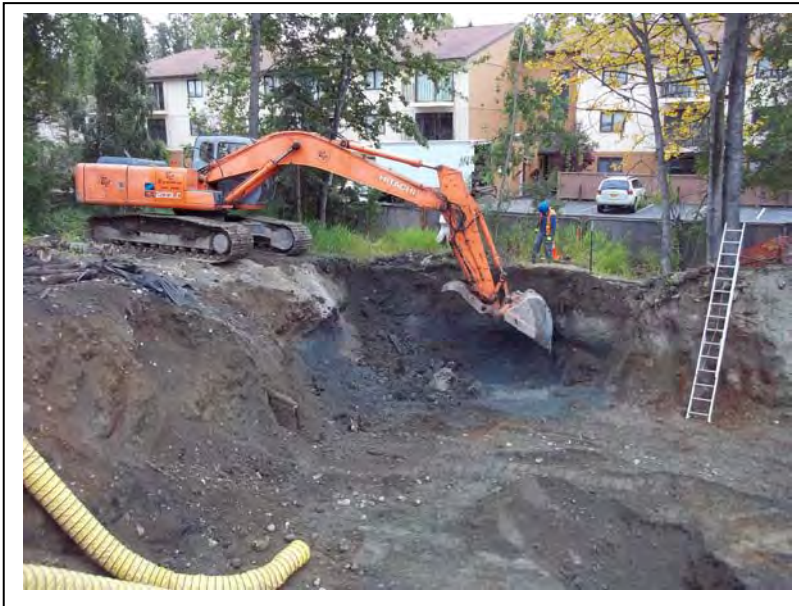
Photo 17: Facing southeast, BCX is conducting the targeted additional excavation. Gray ash-like material indicative of impacted soil is below the excavator bucket. (9/7/2011)
