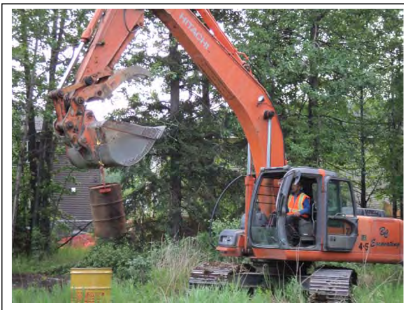
Photo 2: The drum with liquid contents (Drum 1) was placed in an overpack drum. (6/9/2011)
