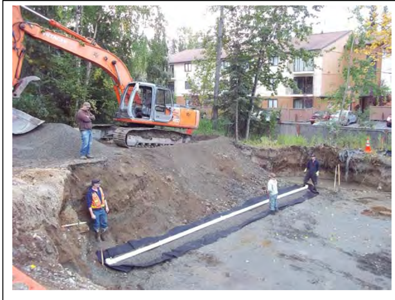
Photo 11: Facing southeast, the deep horizontal vapor extraction piping was bedded in pea gravel and wrapped in geotextile fabric at 10 feet bgs to allow air flow, protect the pipe, and prevent silting.
