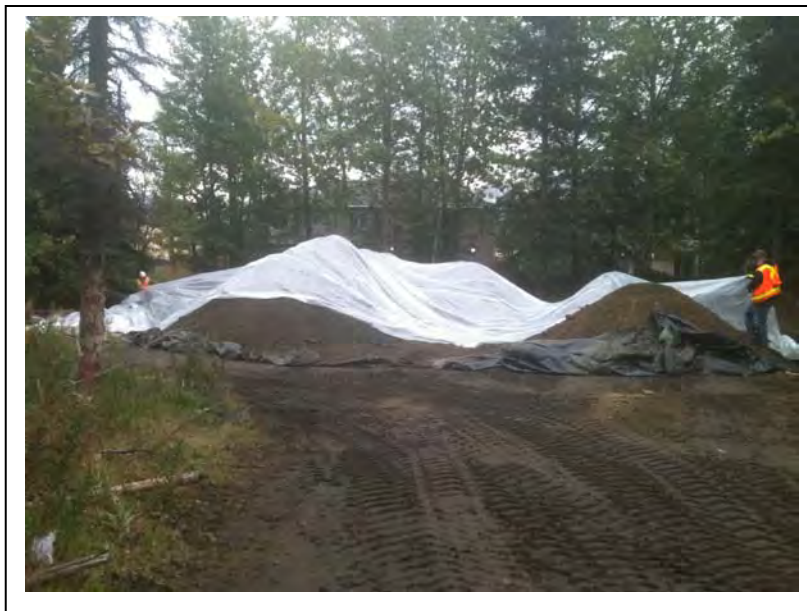
Photo 16: Facing east, BCX removes the 6-mil liner from northeast consolidation area. Soil was segregated in piles, with soil with the lowest screening results (<1 ppm and <5 ppm) in piles on the right. (9/2/2011)
