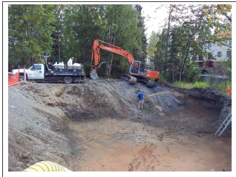
Photo 10: Facing east, a pump on a truck-mounted water tank was used to apply the oxidant mixture to the base of the first lift of the treatment cell. (9/8/2011)
