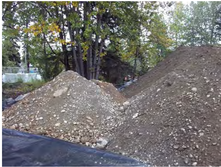
Photo 15: Facing east, the north consolidation area is shown, with the soil pile with >1,000 ppm screening results on the left, and soil with <100 ppm screening results on the right. (9/6/2011)
