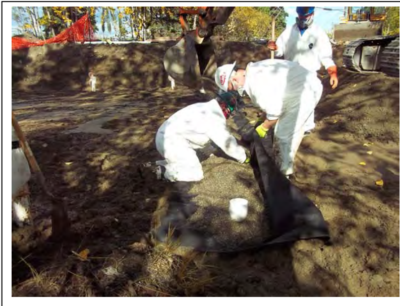
Photo 13: Facing north, the vapor horizontal vapor extraction system components include a 4-inch slotted PVC pipe which was bedded in pea gravel and enclosed in a geotextile. (9/13/2011)
