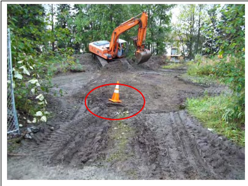
Photo 3: Facing south, the location of the potentially-damaged Monitoring Well MW16 is circled. (9/1/2011)
