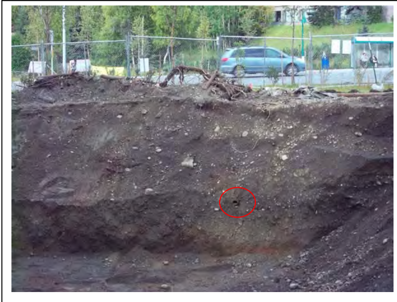
Photo 19: Facing west, the location of the bituminous fiber pipe on the west wall of the excavation is circled. (9/7/2011)
